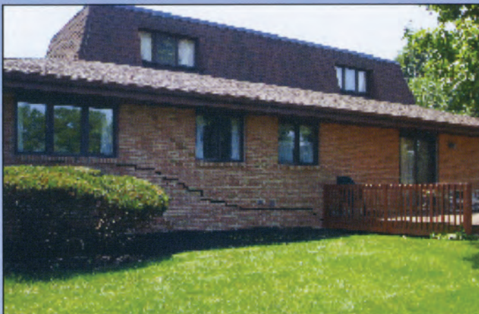
Cracked brick siding as a result of the home dropping into the ground.
