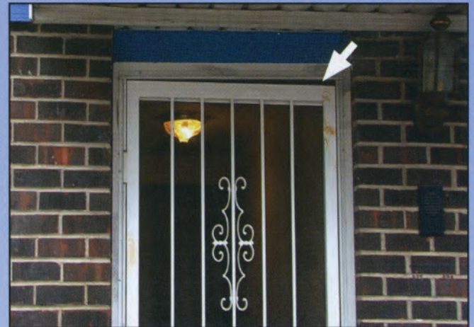
Doors drop due to foundation settling.
