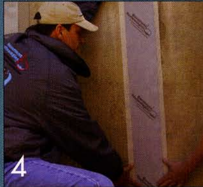
4 We apply a Hydrophobic Gel on the back of the Techni-Crack membrane and apply it to the wall, then tie it into the Water Trek Aqua Route® system or drywell.
