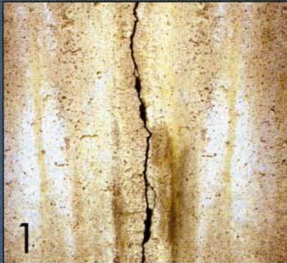
1 Poured foundation wall cracks generate water onto your floor.
